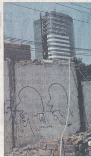
Zhang's graffiti art was drawn on buildings being razed to build Beijing's skyscrapers.
